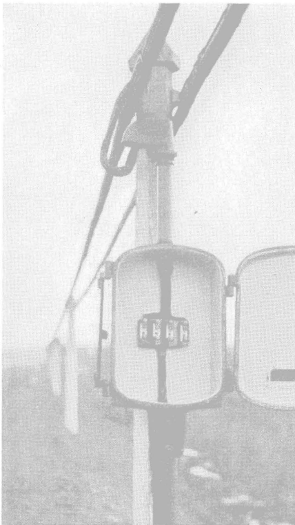
Aerial cables are run on concrete posts
